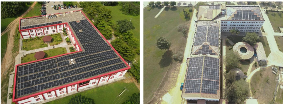
Fig. 6. Aerial view of the roof-top PV solar system.
