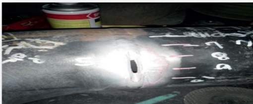
Figure 11: Pipeline Showing Crack with Measurement (Source adapted from [15])
